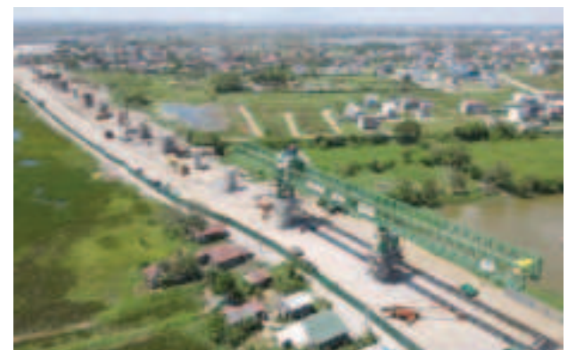
RAILWAY CONSTRUCTION. The launching gantry dubbed “Luid” used in the construction of the North-South Commuter Railway (NSCR) Malolos-Clark segment in this undated photo. Acting Transportation Secretary Giovanni Lopez said Thursday (May 28, 2026) that more than 31,000 jobs for Filipinos have been generated by the NSCR and the Metro Manila Subway Project. (Photo courtesy of DOTr)
