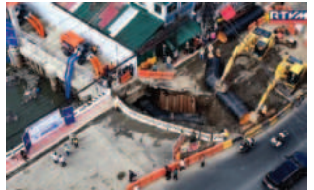
FLOOD MITIGATION. President Ferdinand R. Marcos Jr. inspects the G. Araneta Drainage Improvement Project in Quezon City Wednesday (May 20, 2026). The over PHP482-million, 758-meters long project is targeted to be completed by May 31, 2026. (RTVM screengrab)
