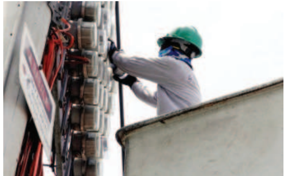
REFUND. A Manila Electric Co. (Meralco) worker conducts a routine inspection of overhead power meters along Road 10 in Tondo, Manila on April 23, 2026. Senator Bam Aquino said Tuesday (April 28, 2026) that electricity subsidies and mandated discounts should be funded through the national budget instead of being passed on to consumers. (PNA photo by Yancy Lim)
