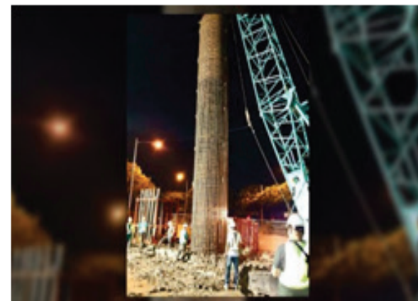
RIGHT-OF-WAY. Piling works of the LRT-1 Cavite Extension. According to the LRTA, the delivery of the right-of-way of the project is almost complete with one pipe from Maynilad, telecommunications (telco) and cable facilities of six companies, and 18 lots of three landowners remaining. (Photo courtesy of DOTr-LRTA)
