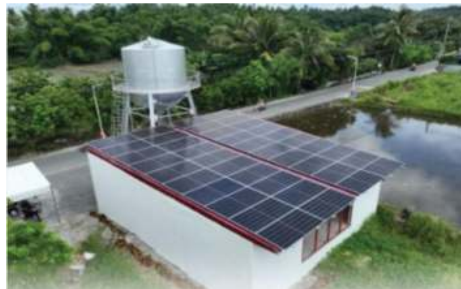
SOLAR-POWERED WATER SYSTEM. A solar-powered water system built by the Department of Public Works and Highways (DPWH) in Barangay San Guillermo, Lipa City, Batangas province. Similar projects were built by the agency in Barangay Castillo, Padre Garcia town, and Barangay Catandala in Ibaan. (Photo courtesy of DPWH Batangas 4th DEO)
