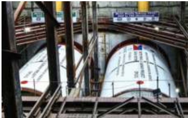
Construction of Metro Manila Subway Project in Quezon City (PNA file photo by Joan Bon-doc)
