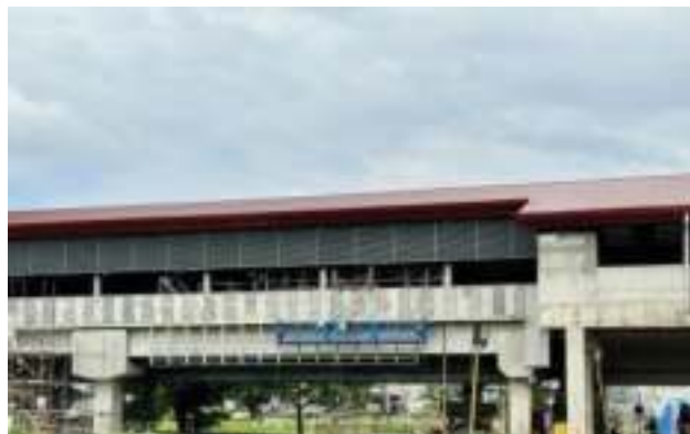
NEARING COMPLETION. The under-construction Dr. Santos Station of the Light Rail Transit Line 1 (LRT-1) Cavite Extension in Parañaque City in this undated photo. The Light Rail Manila Corp. said Wednesday (March 6, 2024) that the first phase of the Cavite Extension project is 97 percent complete and will be operational by the fourth quarter of 2024. (Photo courtesy of LRMC)
