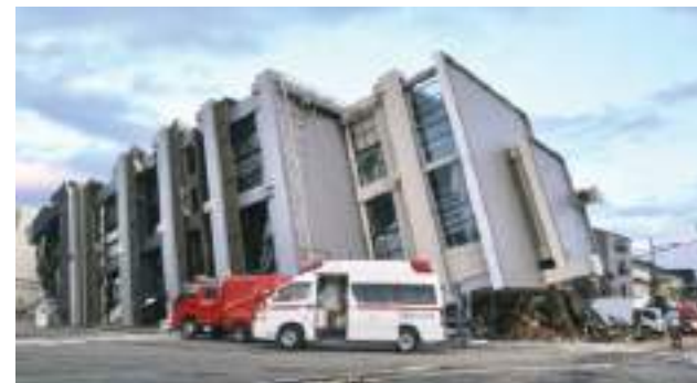
QUAKE DAMAGE. A collapsed building in Wajima City in Japan's Ishikawa Prefecture on Jan. 2, 2024. The DFA said no Filipino was among the eight reported casualties in the massive earthquake that struck central Japan on New Year's Day (Jan. 1). (Kyodo photo)
